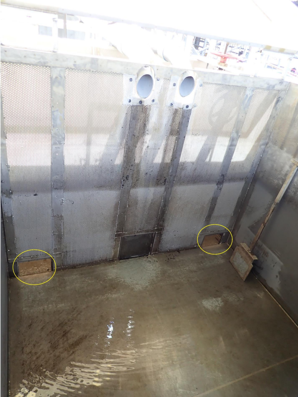
Image 2: Missing perforated screens in sample tank "B".
